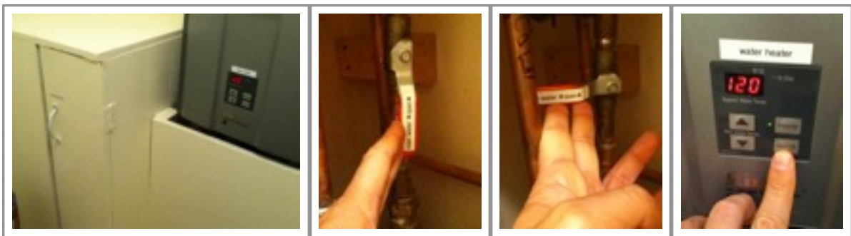
(from left to right) View of the water heater to the right of the access door for the main water valve. Main water valve rotated counter-clockwise into open position. Main water valve rotated clockwise into closed position. Water heater “on/off” button being pushed (water heater currently “on” and set to 120 degrees).
